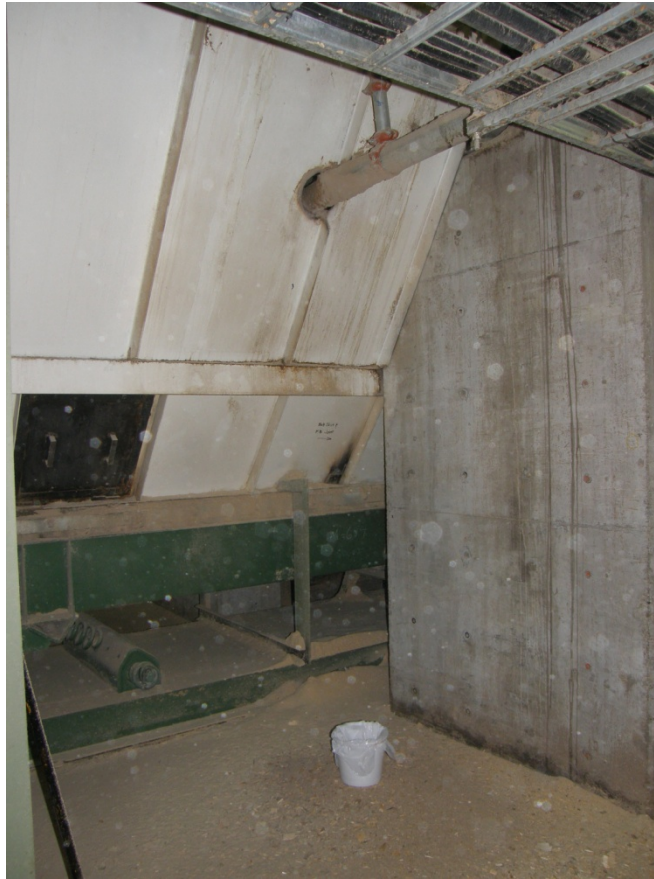
Figure 19 Sawdust on basement floor due to unsealed opening in the conveyor chute
