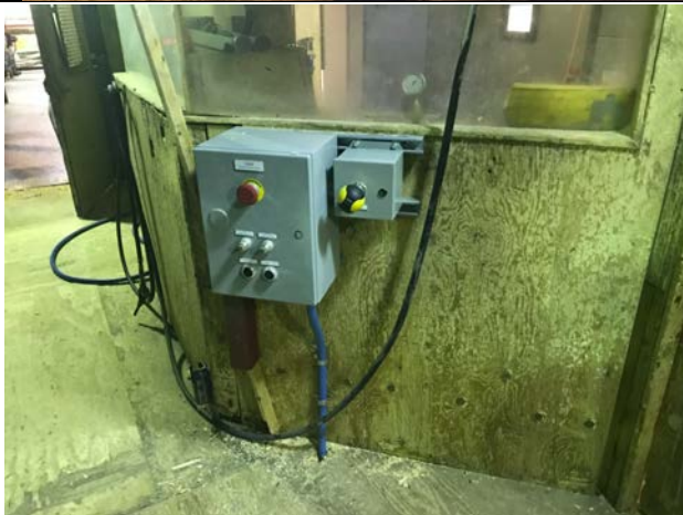
This is the manual control panel on the inside of the planer room. The panel is used when jointing mode (mode 3) is entered whereby the millwright must select and acknowledge the mode change, remove the jointing key from the CS02 panel, and insert the key into one of the jointing key switches shown here. This then allows the top or bottom head (one or the other) to be jointed.
