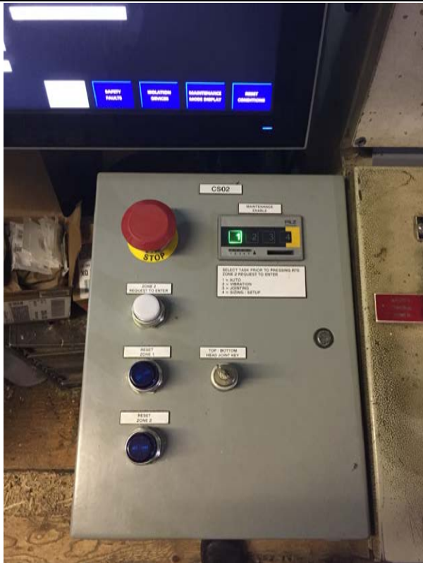
CS02 safety system operation panel at main planer entrance (zone 2).
